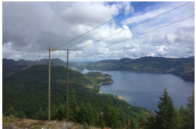
A BC Hydro transmission line near Upper Campbell Lake
