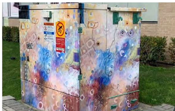
The Town of Sidney added decorative wraps to BC Hydro equipment in their community.
