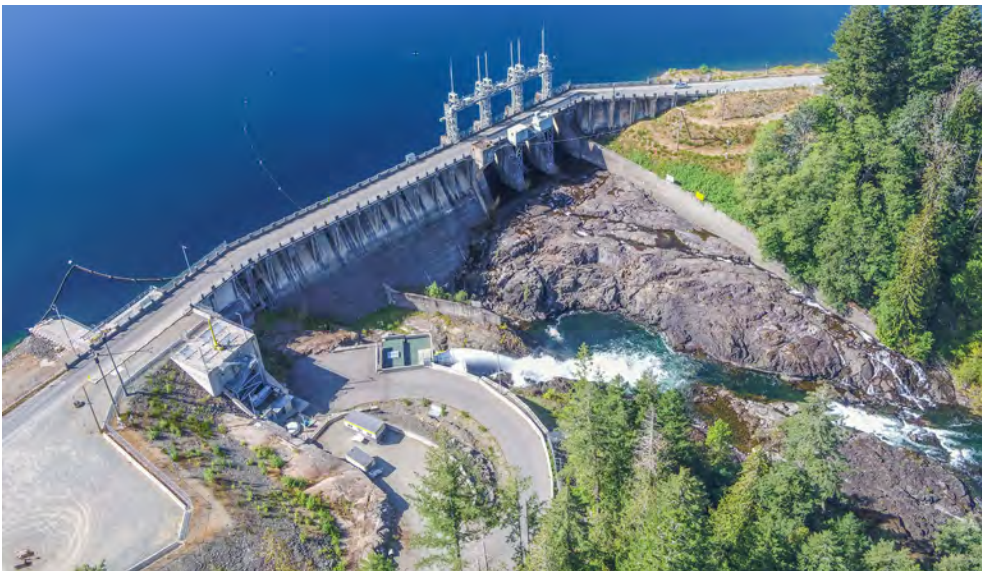
Site work has begun to prepare the area around the John Hart Dam in Campbell River for the upcoming John Hart Dam Seismic Upgrade Project. The Project includes seismic upgrades to strengthen the dam so it can withstand a severe earthquake. For more information on this project, as well as the Ladore and Strathcona projects, visit majorprojects.ca
