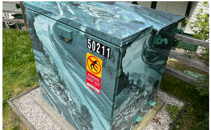
Example of a decorative wrap on our pad-mounted equipment.
