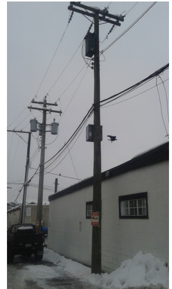
Power supply photo sample
